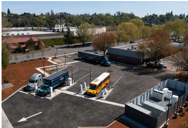
Figure 28: Heavy-Duty Electric Charging Station in Portland, OR
